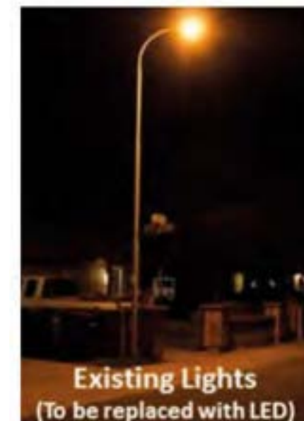
Existing 2200 Kelvin HPS
