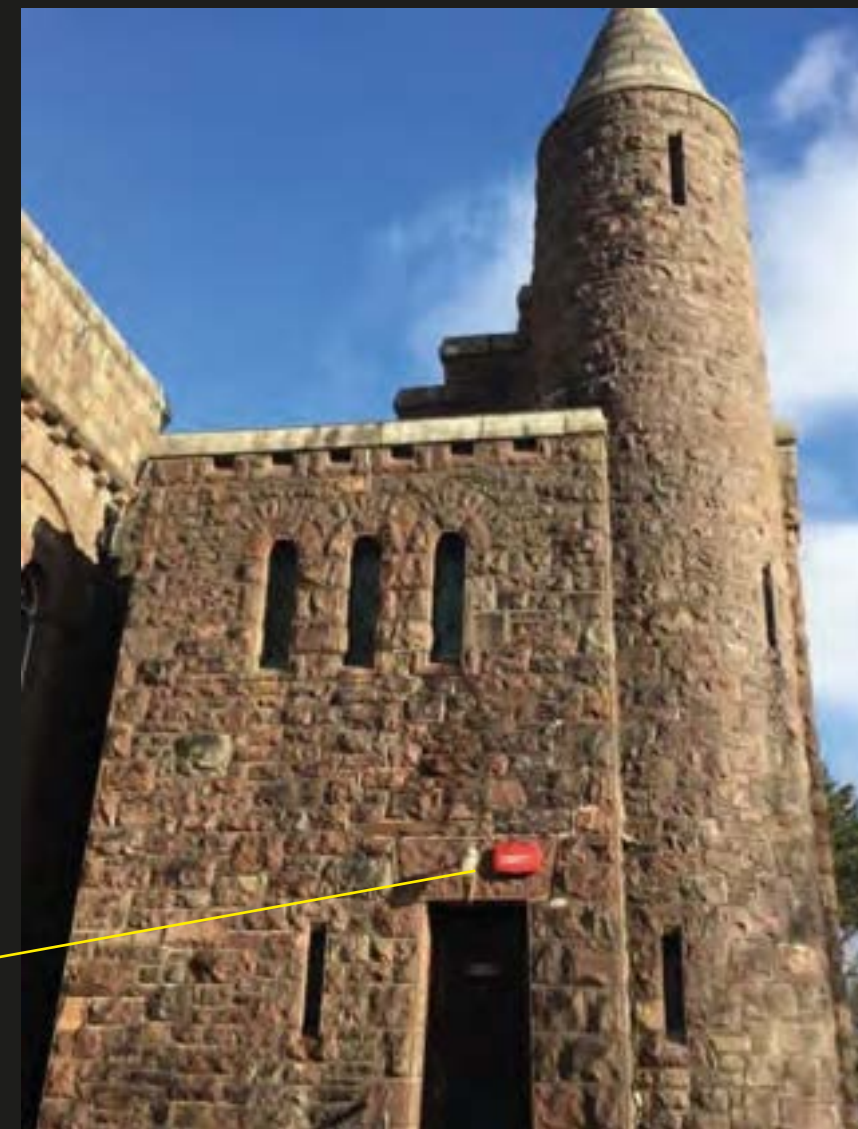
New cut-off lighting for the entrances.
